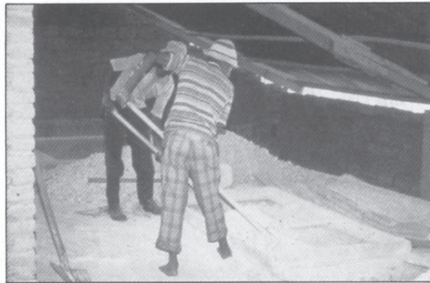
The lime production line.
