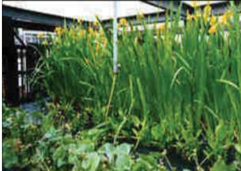
FIGURE 5.6.21 Grey water treatment roof
