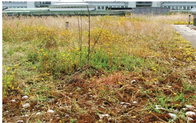
FIGURE 5.6.19 Biodiverse vegetation established from seed on a low-nutrient lightweight substrate to a roof in Basel
